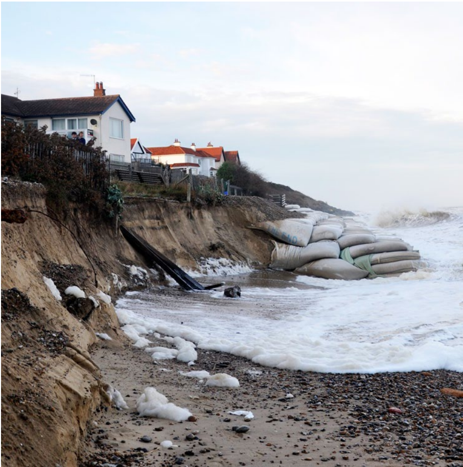
5. Thorpeness, showing cliff erosion. (Photo: Fran Crowe.)
